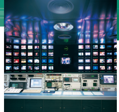
Digital network operations room for the monitoring of the transmission function of TV satellites. Photo: SES
